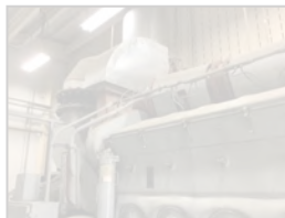
EMD DIESEL ENGINE-GENERATOR SYSTEM MODEL: EMD-20645E4B 900 RPM; Continuous Duty; 2200 KW, 480 Volt, 3 phase, 60 hertz; Turbo-Charged; Skid Mounted S/N: 82-2-1035
